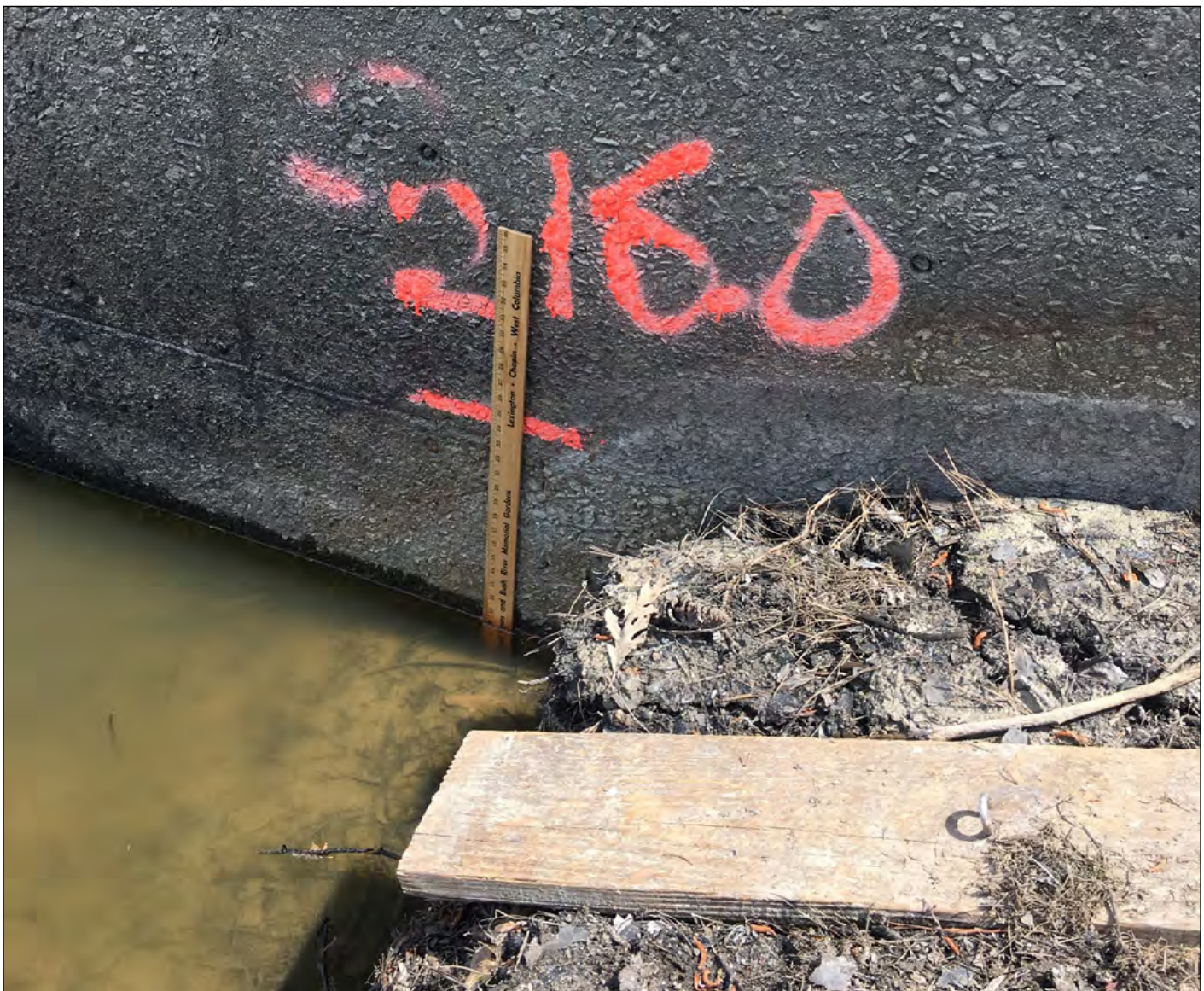
Figure 4 Springwood Lake Dam Auxiliary Spillway Marked With the "Safe" Water Level Elevation of 216.0-ft MSL (NAVD88)
